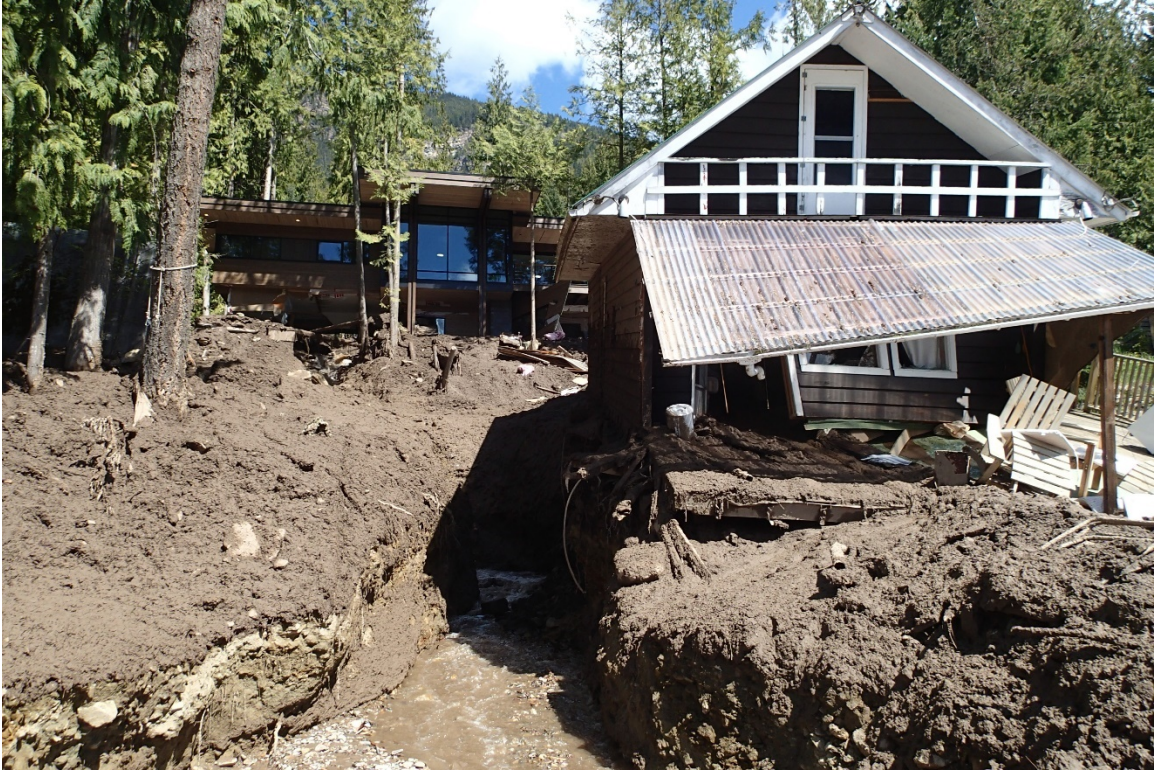
Figure 1-4. Damaged buildings from the 2017 Robinson Creek debris flow. Photo: BGC, May 7, 2017.
